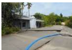
(園路の被災状況)
